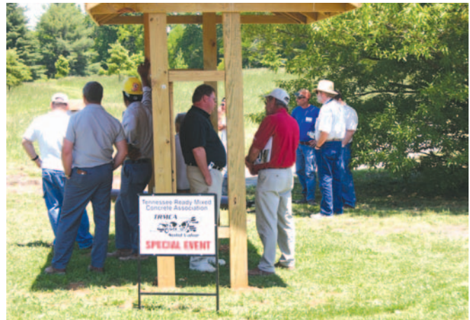
Interested observers gather at Henry Horton State Park to watch the first section of a new pervious concrete walking trail be installed, thanks to donations of labor and materials by TCA members.
