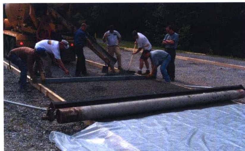
Erwin demo project constructed through a collaborative effort with TVA grant money, the Appalachian RC&D Council, and TRMCA. Transit Mix and Loven Ready Mix donated some pervious concrete, and Watauga Ready Mix donated the use of the roller.
