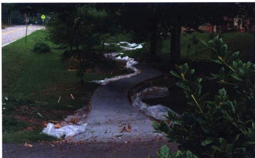
On this Knoxville sidewalk, pervious concrete allows water to pass through, irrigating surrounding foliage. Project completed as a donation by TRMCA, with concrete provided by American Limestone and Ready Mix of Knoxville.
